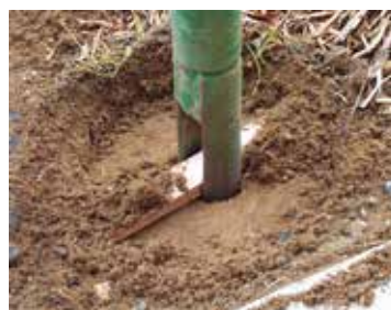
Photo 4. A piece of wood in the auger channel helps clear the soil surface to create a flat base for the Sentricon station. It may also be used to clear lawn, gravel or mulch.
